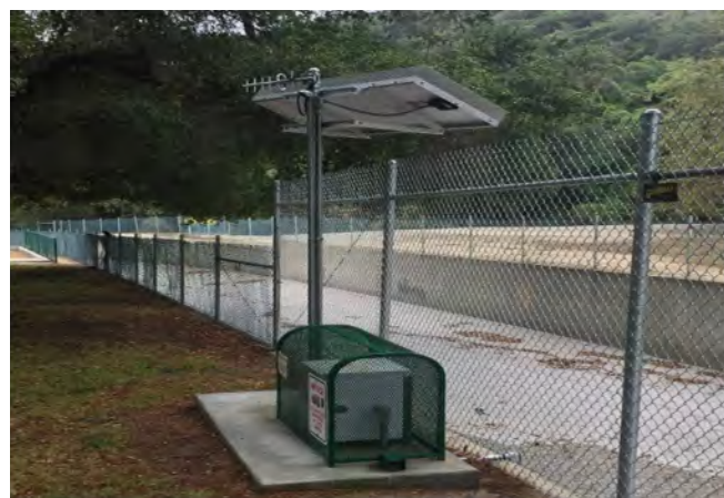
Flow Monitoring Station 1- Verdugo Wash Upgradient
