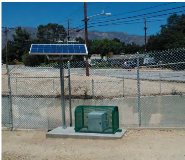
Flow Monitoring Station 2- Verdugo Wash Downgradient
