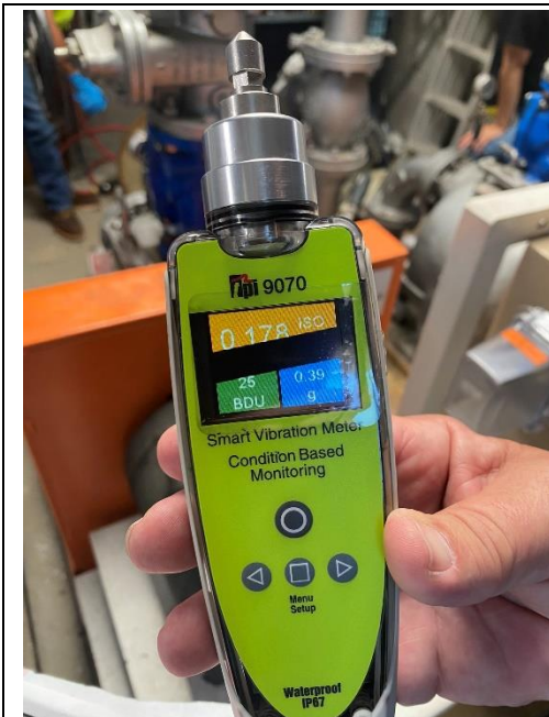
Figure 9: Pump 1 Vibration Meter
