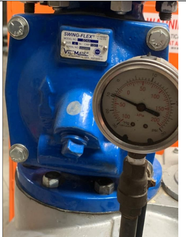
Figure 12: Suction Pressure Gauge
