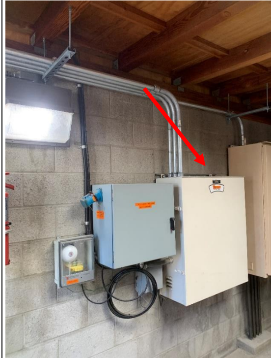
Figure 20: Control Panel Location
