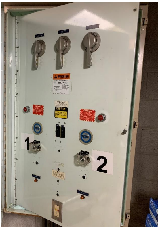
Figure 30: MCC Internal Panel
