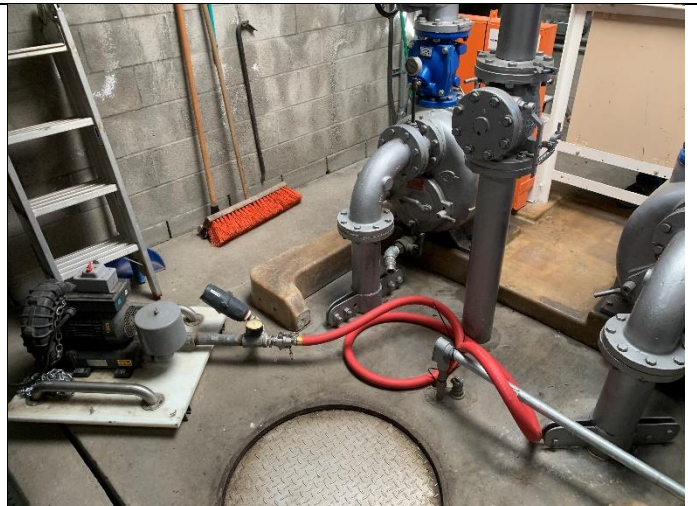
Figure 2: Manhole, Blower, and Suction end of Pumps
