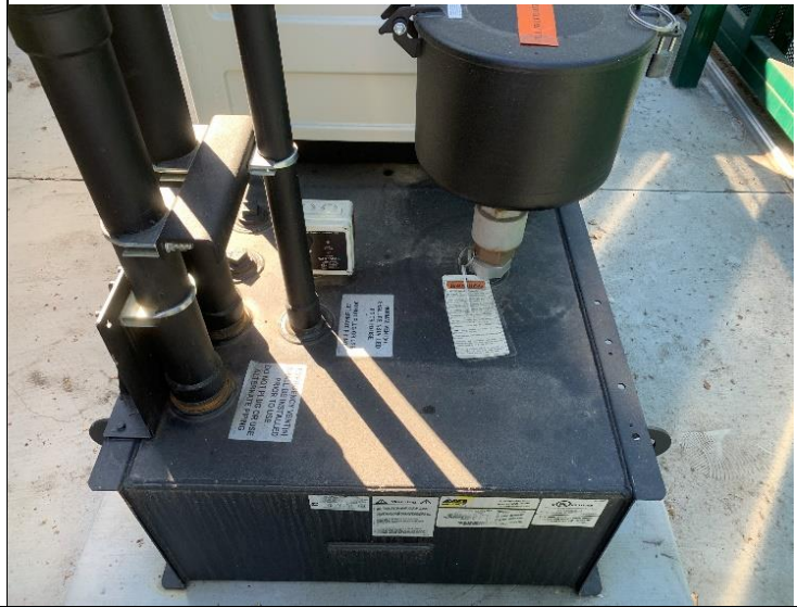
Figure 39: Generator Fuel Tank
