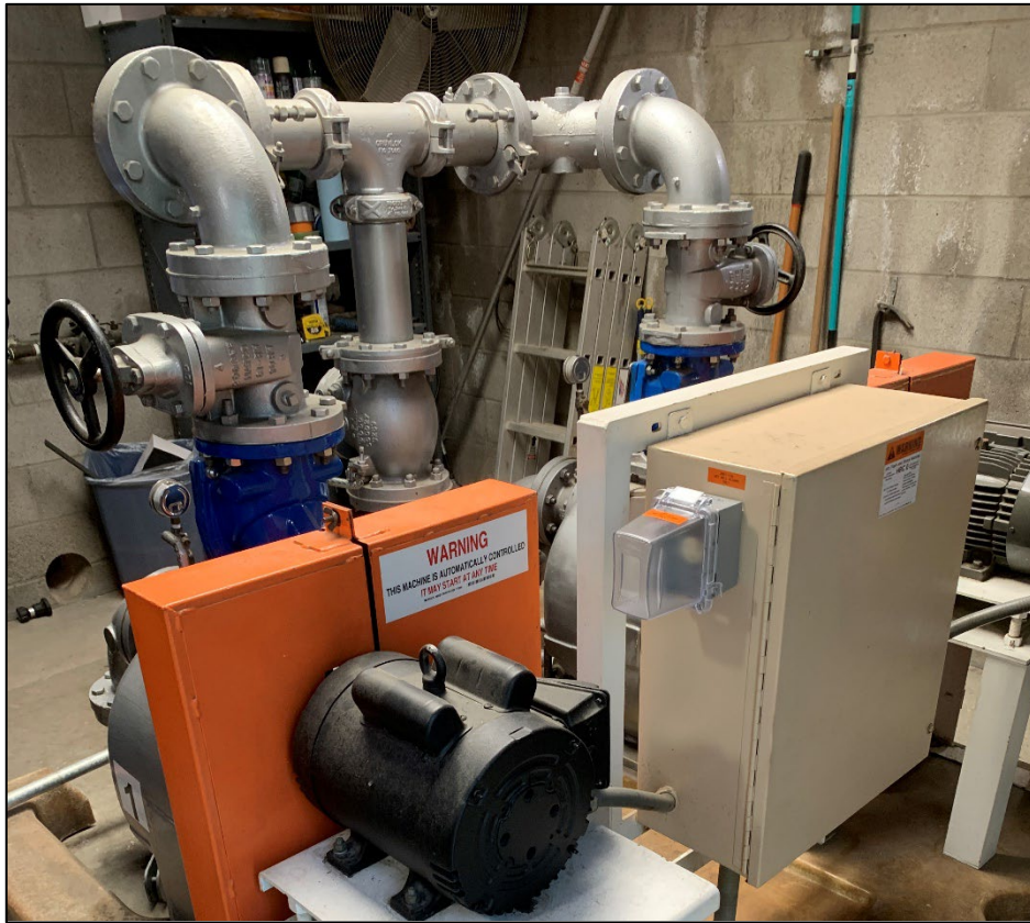
Figure 5-11: Lift Station Discharge Header
