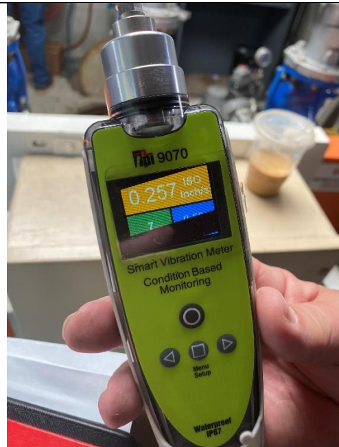
Figure 10: Pump 2 Vibration Meter
