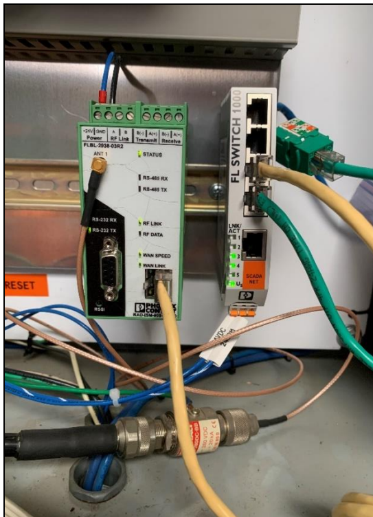
Figure 36: SCADA Hookup – Appears to be hooked up to Coaxial here
