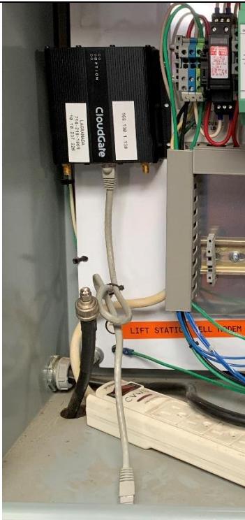
Figure 34: Cloudgate SCADA Modem – not hooked up?
