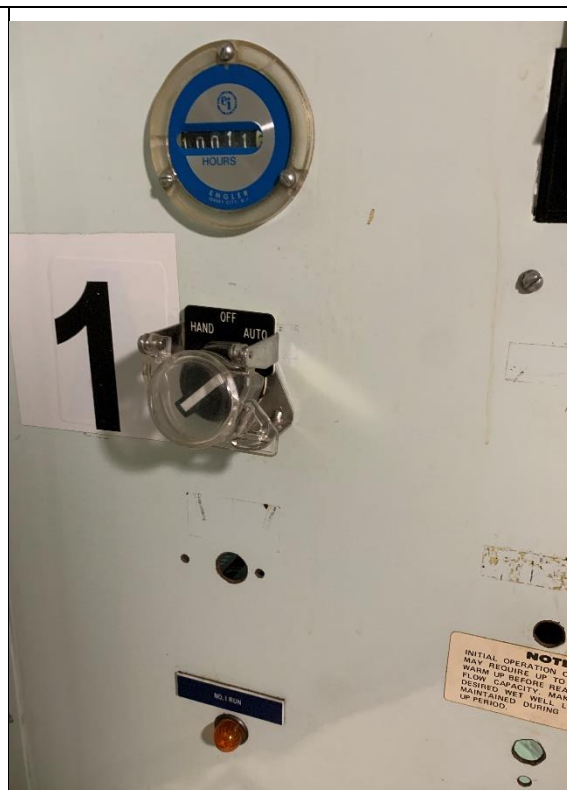
Figure 31: MCC Internal Panel HOA and Runtime
