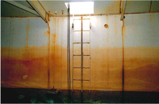
Edmund No. 2 – 2020 Severe Corrosion
