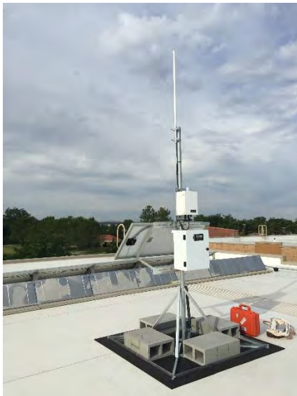
Floor-Mounted Collector with Solar Panels
