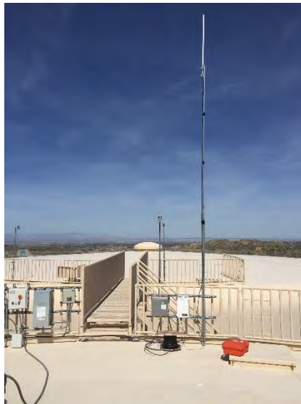
Tank Rail-Mounted Collector with Long Mast
