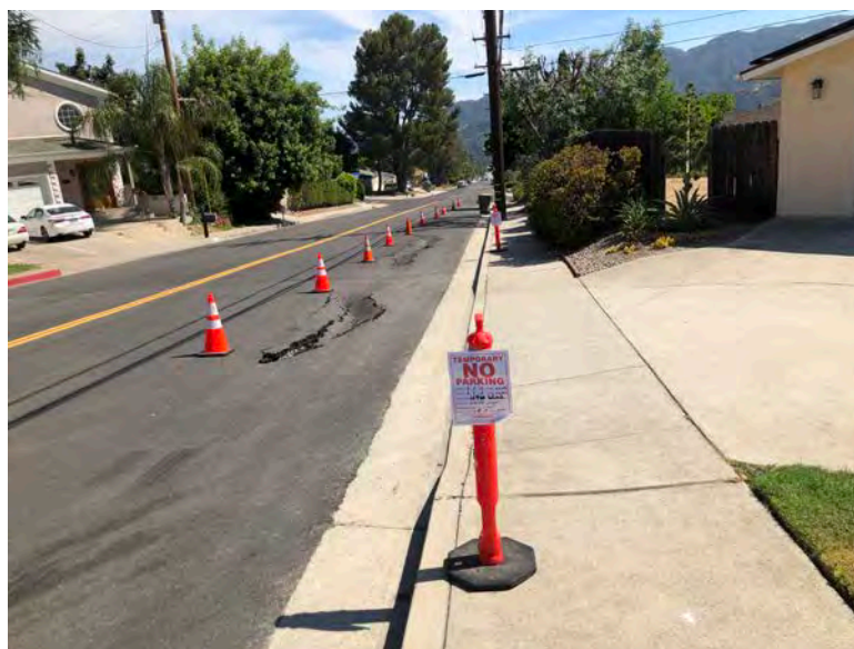
Pavement Damage – Looking South
