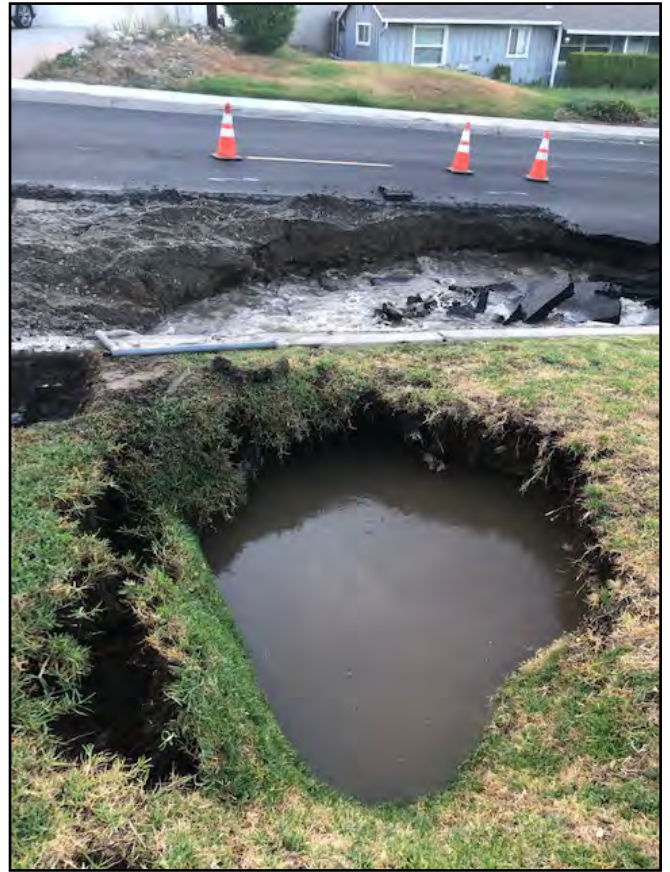
Leak in front of 4811 Pennsylvania
