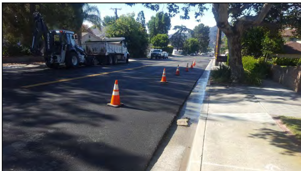
Pavement uplifting at edge of gutter
