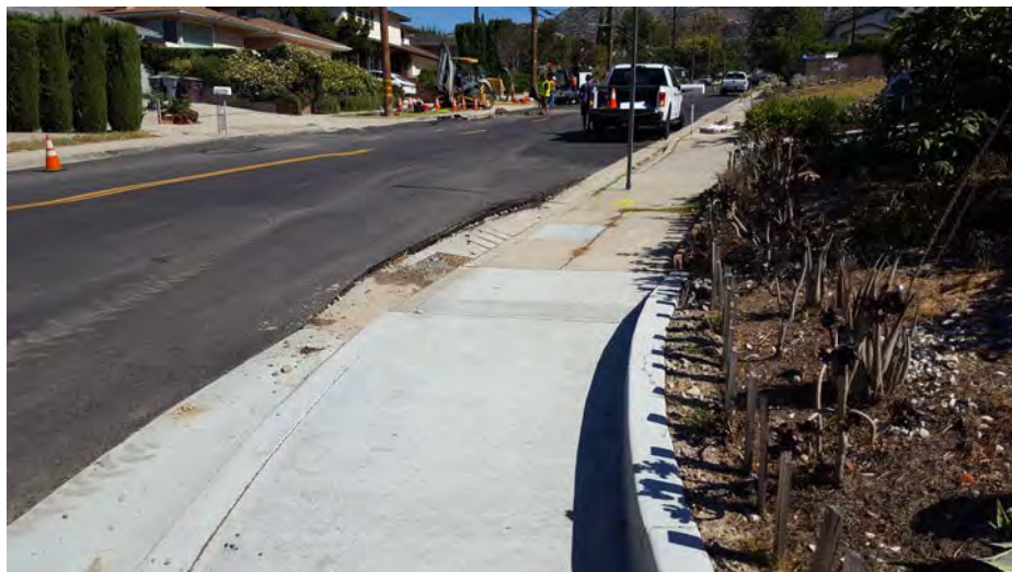
Pavement uplifting at Penn. & Stevens – Looking North
