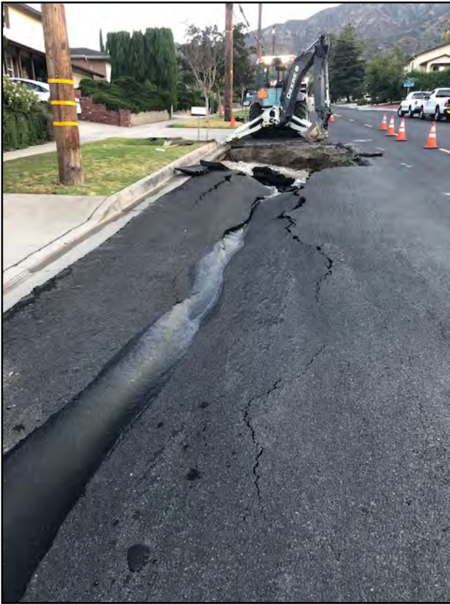
Main Break – Pennsylvania Ave – Looking North
