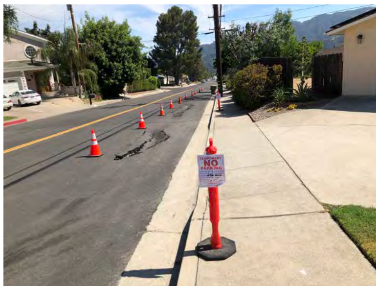
Pavement Damage – Looking South
