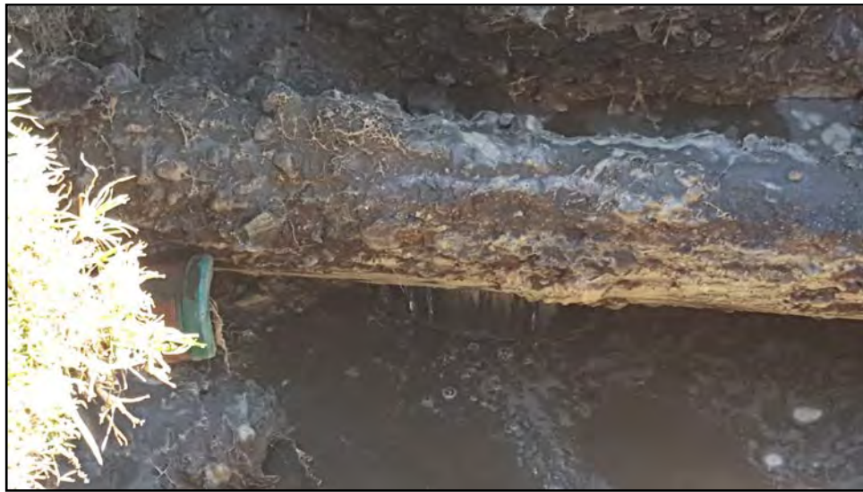
8-inch Pipeline – Leak on bottom of pipe and 4-inch Sewer Lateral
