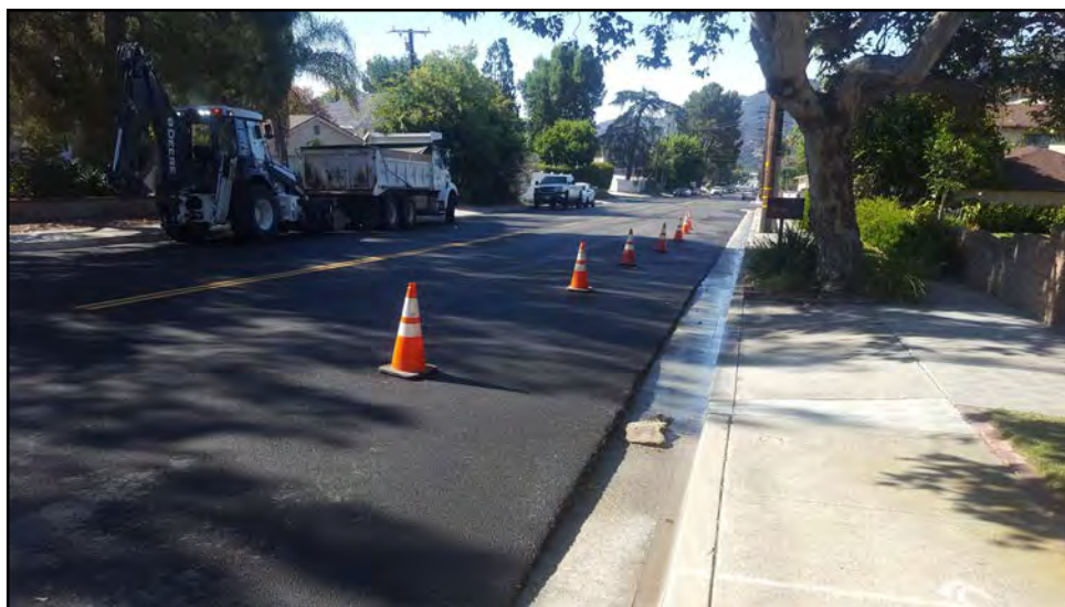
Pavement uplifting at edge of gutter
