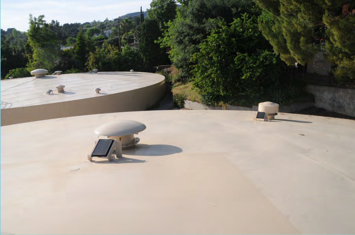
Oak Creek No. 1 & No. 2 – Exterior Solar Power Roof Fans
