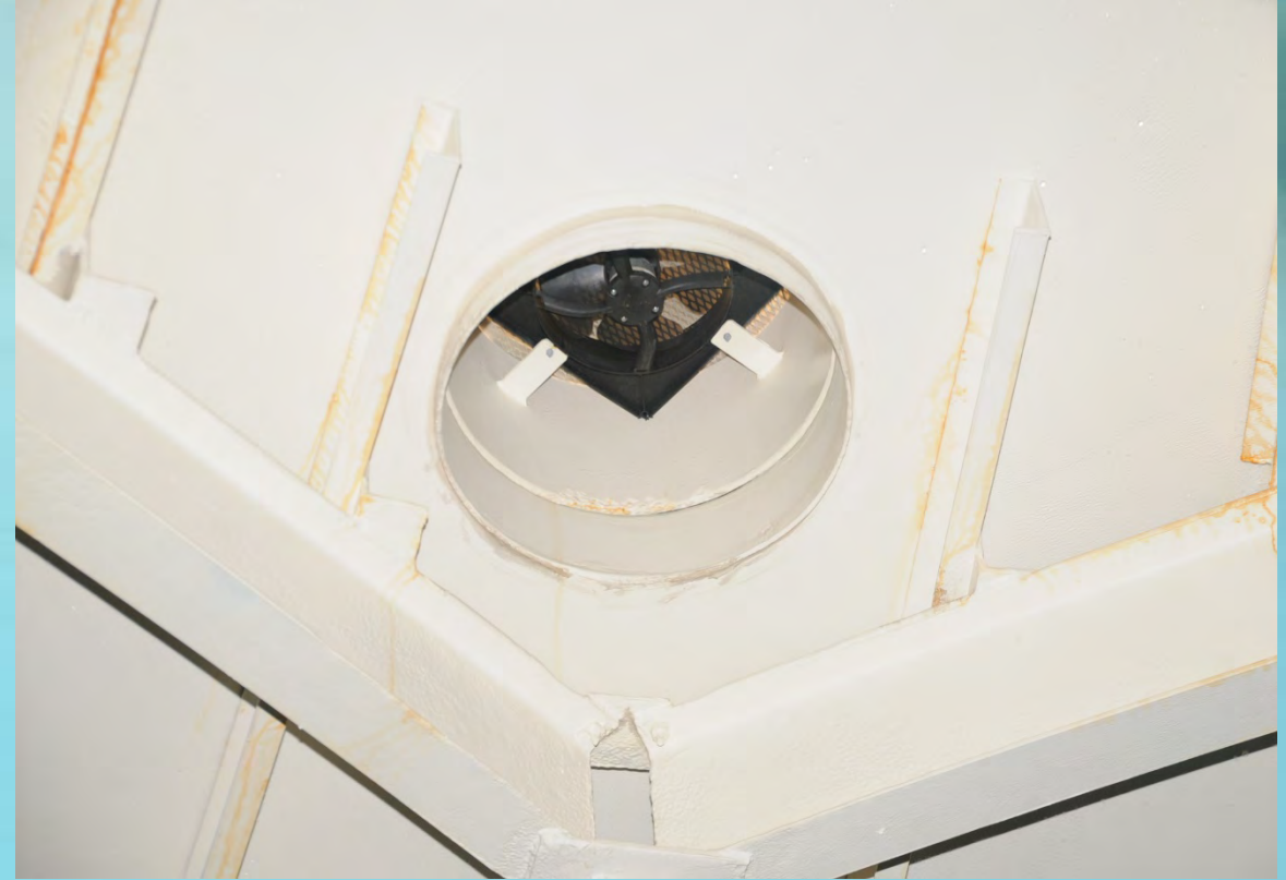
Oak Creek No. 1 – Interior Solar Power Roof Fan
