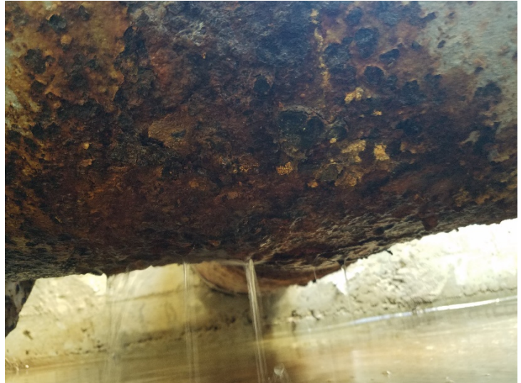
Figure 2 - Bottom of manifold. Source of the leak. Pipe not suitable to weld.
