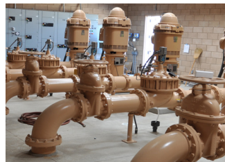
Pump Station and PRS
