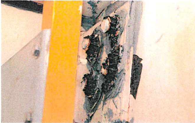
Goss Canyon No. 1 – 2015 Severe Corrosion gusset plate connector
