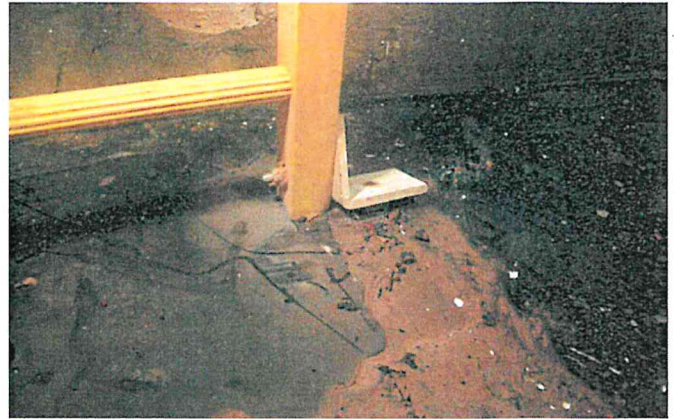
Goss Canyon No. 1 – 2015 Anchor bolt missing at Ladder
