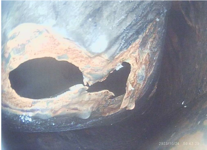
Figure 2: Bore Inspection Snapshot of Leak
