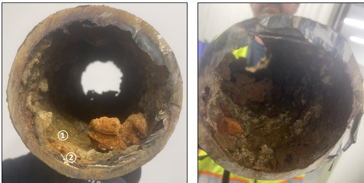
Figure 15 – Internal Corrosion of an Unlined Iron Pipe Removed from the Corner of Cecilville Avenue and Orange Avenue
