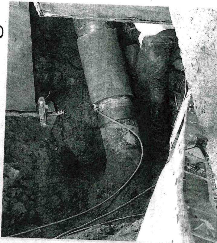
Photos by Anne McNEILL Breaks in aging water mains, like this one that occurred on May 31 on Pennsylvania and Henrietta avenues, is a reason that CVWD is considering a capital charge on the property tax roll.
