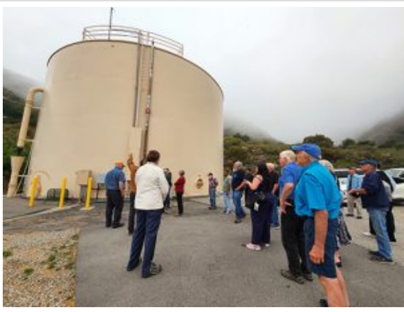
A water tank stores treated water manages water flow.
