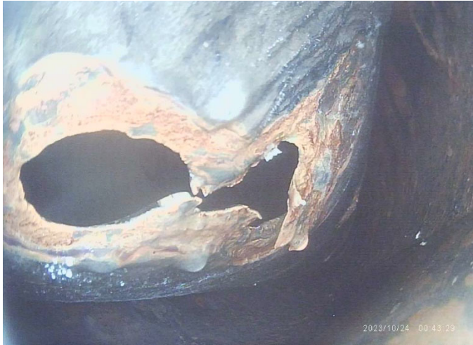
Figure 2: Bore Inspection Snapshot of Leak
